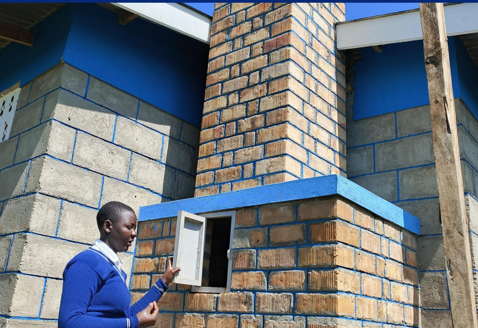
Ruth demonstrates the use of the Incinerator
