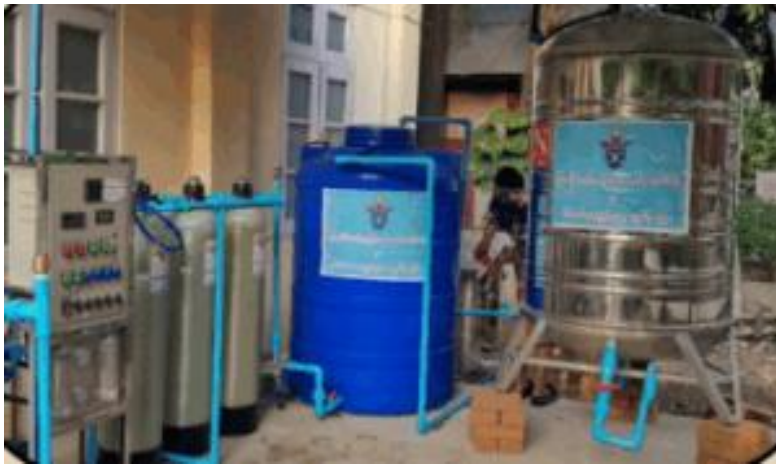
The water purification systems that were installed.
