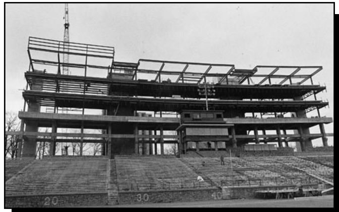
The old press box, which could barely seat 50 members of the media, was dwarfed by construction of the new press tower.
