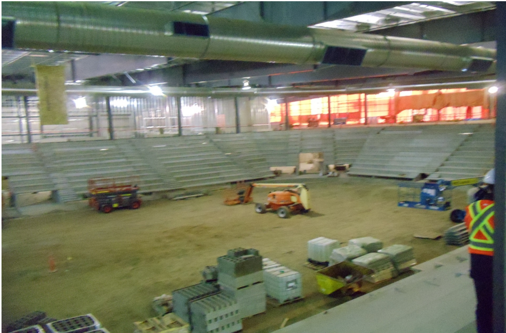
On 4 June 2018 the interior work had reached more than 50% completion. Photograph by M.P.J. Kennedy.
