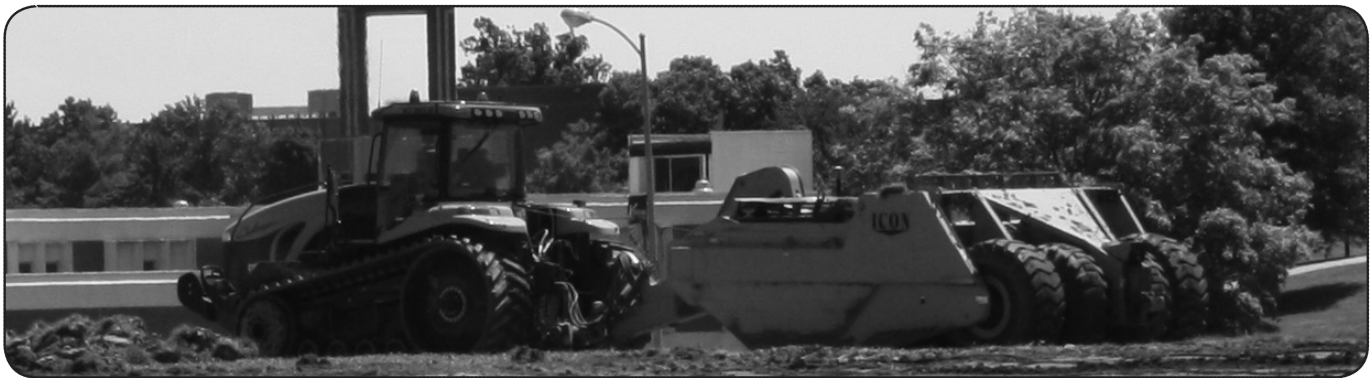
Heavy dirt work takes place on the construction site. The indoor facility will sit on the site directly in front of Spratt Stadium which was formerly the home of the MWSU Softball Complex. The main portion of the facility will sit on the area formerly occupied by Field Two, while a new 300-space parking lot will occupy the space where the main game field used to be.
