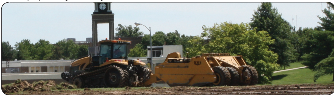
Heavy dirt work takes place on the construction site. The indoor facility will sit on the site directly in front of Spratt Stadium which was formerly the home of the MWSU Softball Complex. The main portion of the facility will sit on the area formerly occupied by Field Two, while a new 300-space parking lot will occupy the space where the main game field used to be.
