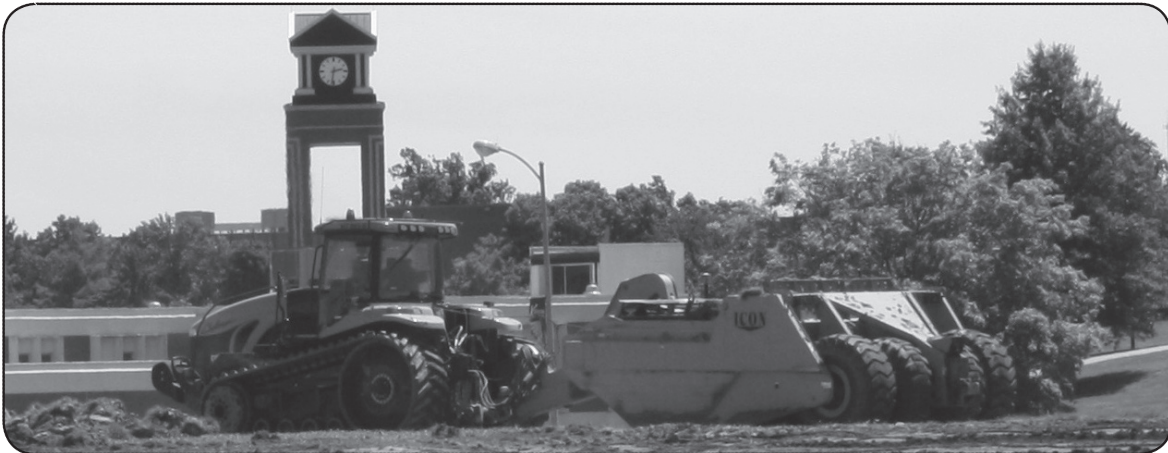
Heavy dirt work takes place on the construction site. The indoor facility will sit on the site directly in front of Spratt Stadium which was formerly the home of the MWSU Softball Complex. The main portion of the facility will sit on the area formerly occupied by Field Two, while a new 300-space parking lot will occupy the space where the main game field used to be.
