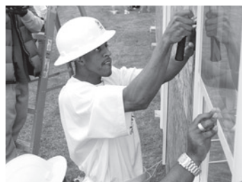
Jerome Williams helps build a Habitat for Humanity house during 2006 All-Star Week in Houston, Texas
