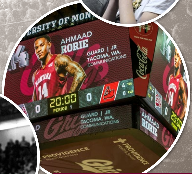
A state-of-the-art video board was installed inside Dahlberg Arena prior to the 2017-18
