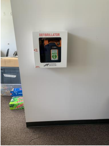
This AED is located inside the Johnson Stadium press box.
