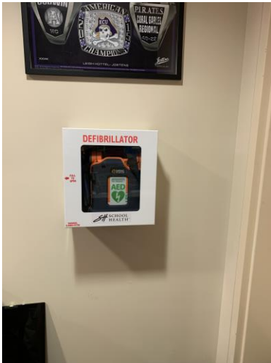
This AED is located in back hallway near the coach's locker room.
