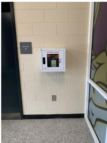
This AED is located in the William – Harvey Team Sports Building on the first floor beside the elevator.
