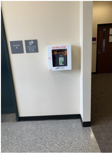
This AED is located in the William – Harvey Team Sports Building on the second floor beside the elevator.
