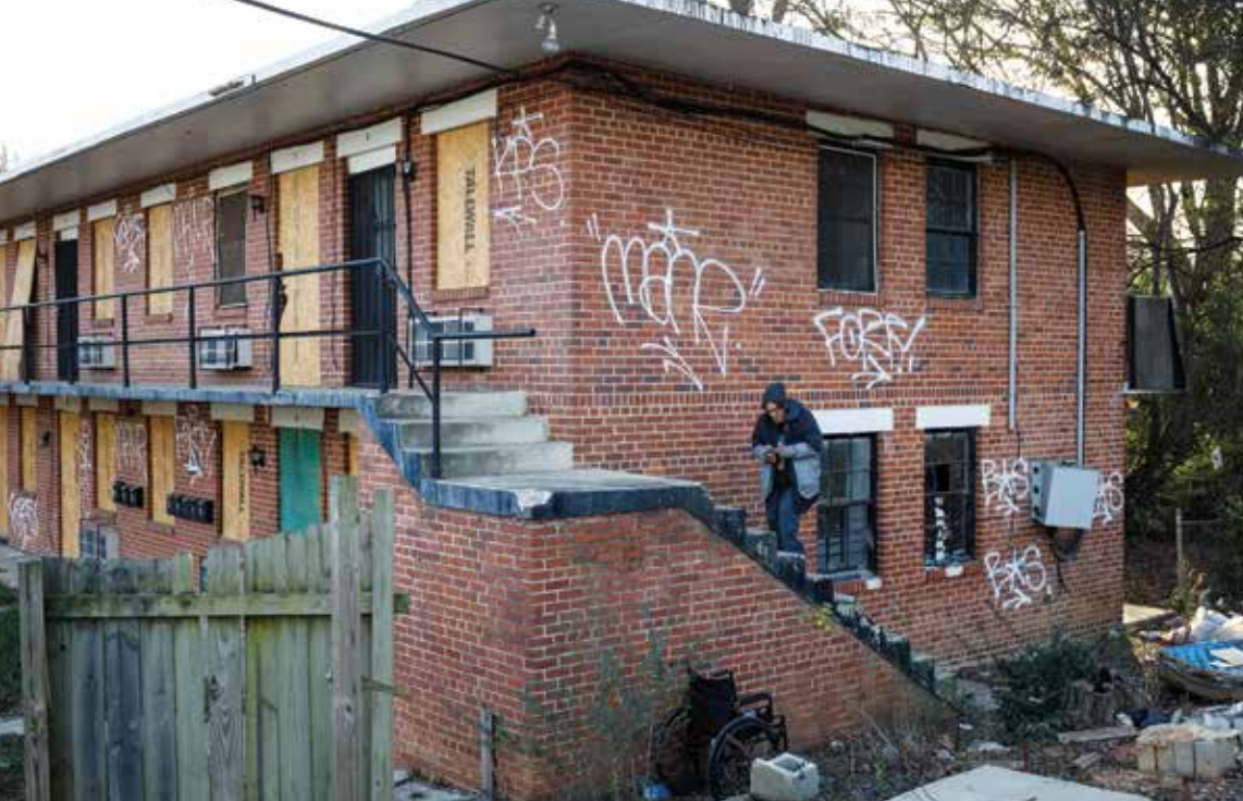
Boarded-up English Avenue apartments became home to squatters like the woman in this photo from 2016.
