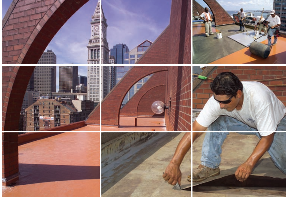
The new Sika Sarnafil membrane installed at the Marriott Long Wharf, Boston, MA. At right, a worker cuts the old membrane, which was recycled and will go back into new membrane production.
