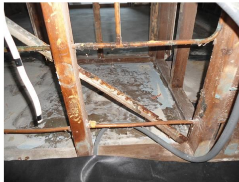
Figure 16: Last time the house was flooded, chlorine or bleach was used to sanitise the frame. As you can see from these photos not only has the chlorine corroded the metal bracing, it was not effective at dealing with the mould spores present on the frame
