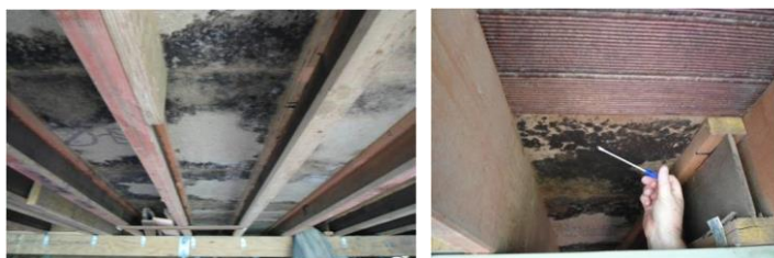
Figure 11: Mould infestation spreading out from joins between particleboard floor sheets and Taking ATP Swab Test
