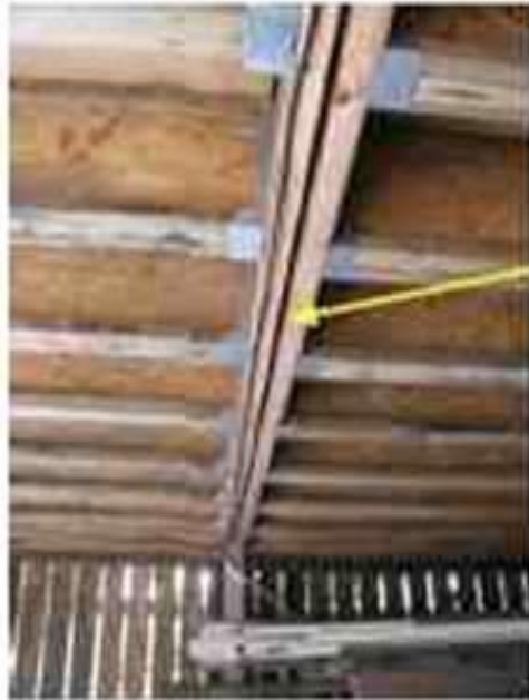
Figure 3: Expansion of the hardwood T&G floor above has caused the separation of double bearers.
