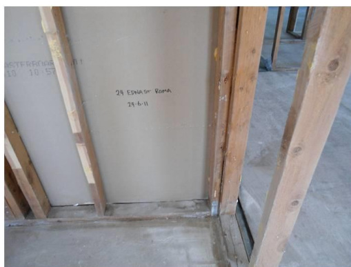
Figure 13: Same house flooded again just over a year later, only difference is after the first flood the timber frame was sanitised by Effective Organics. No mould growth whatsoever in the wall cavity or on the plasterboard.
