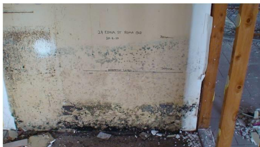
Figure 12: Flooded house in Roma 2010 heavy mould infestation throughout
