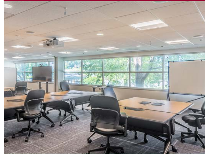
DROP-DOWN LED LIGHTING
