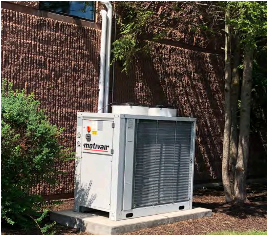
Clean Room Cooling Unit
