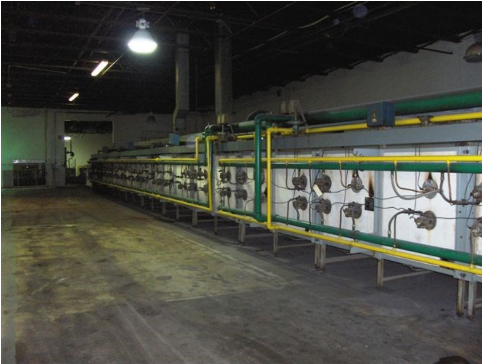
Equipment to be removed
