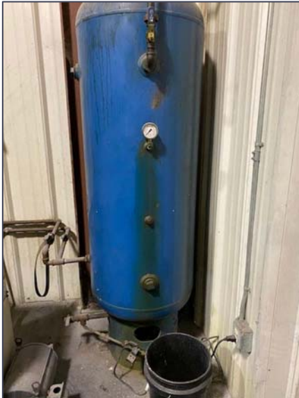
Ingersoll Rand air compressor
