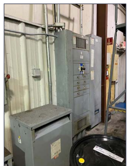
Electric switch gear and transformer
