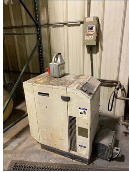
Ingersoll Rand air compressor
