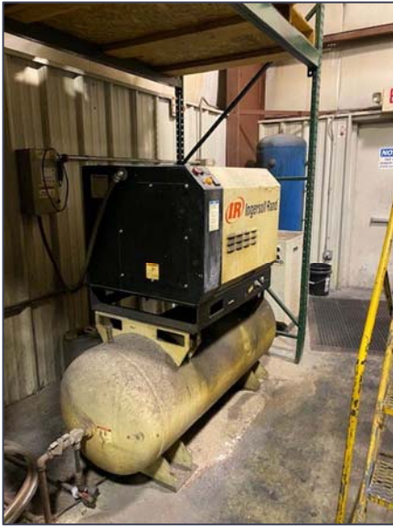
Ingersoll Rand air compressor
