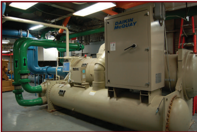
New Chillers in Mechanical Room
