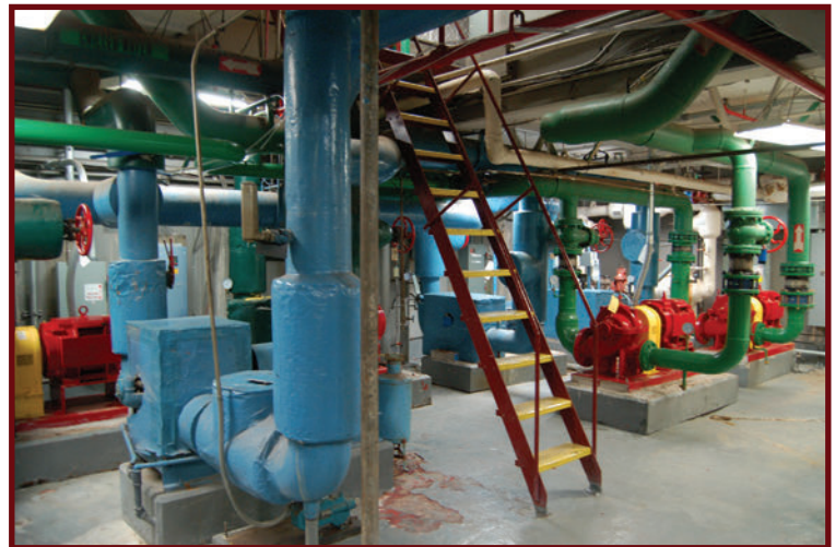
New Pumps in Mechanical Room
