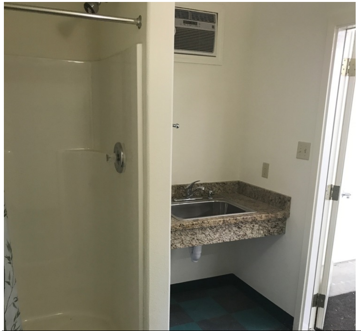
AC, Sink, and Shower
