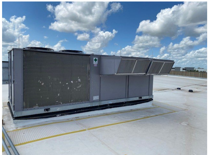
Two 50-ton rooftop units added
