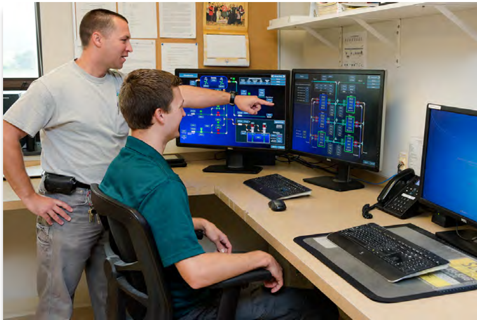
City public works staff monitor real-time information about the operation of the raw water treatment facility
