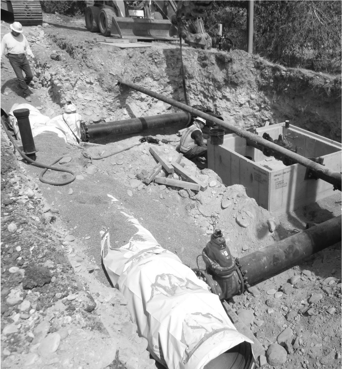
Above Photo – Contractor installing new 24-inch water main in Redlands area. Photo by Tom Ellis.
