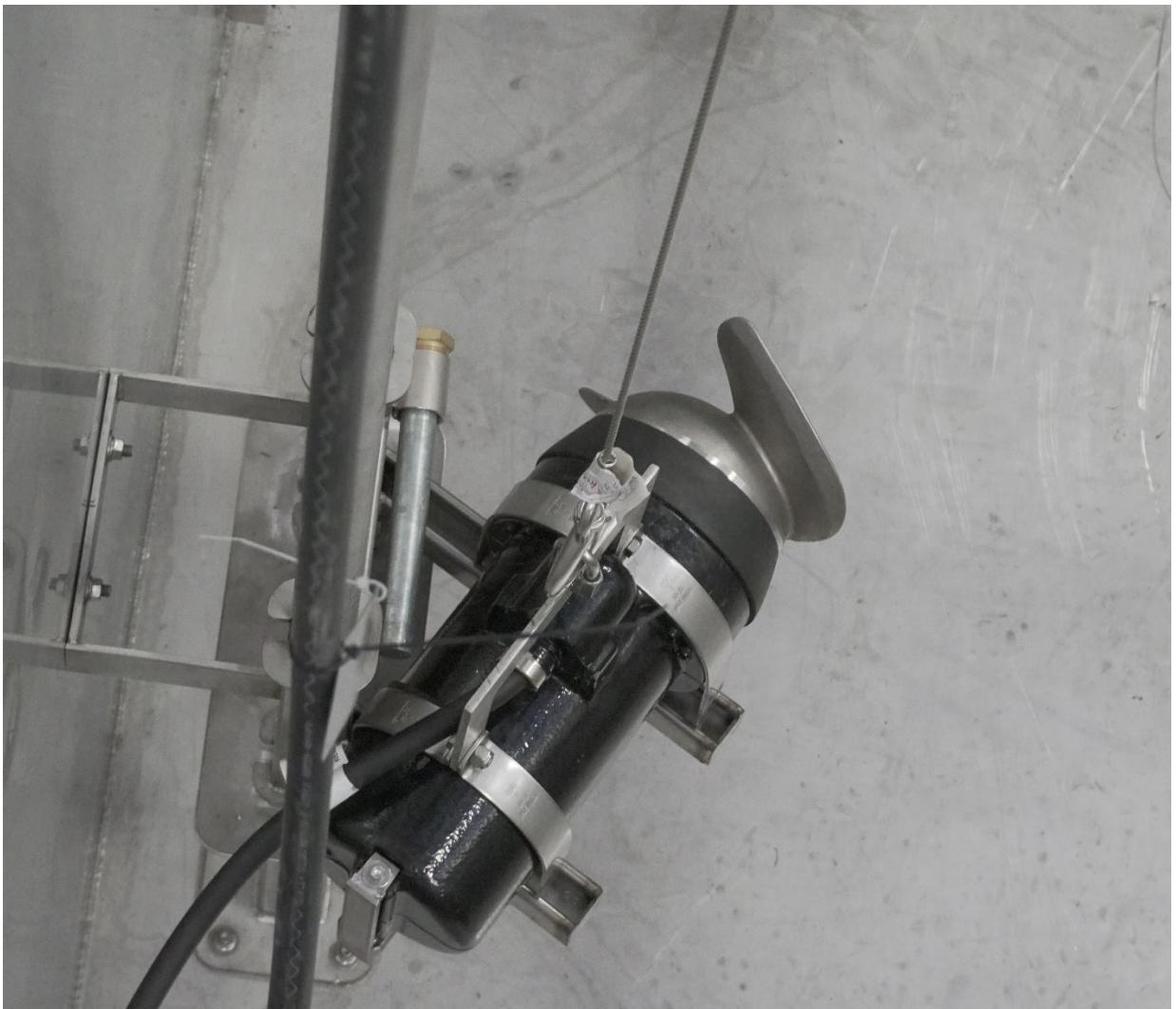
Example Anoxic Mixer Installation
