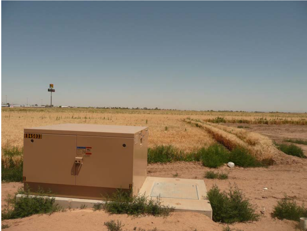
New electrical, view north along Milligan Road of subject site.
