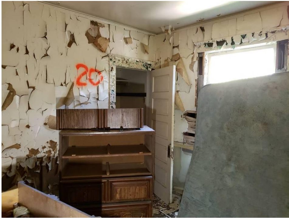
View of FS-20 (2 nd floor unit)
