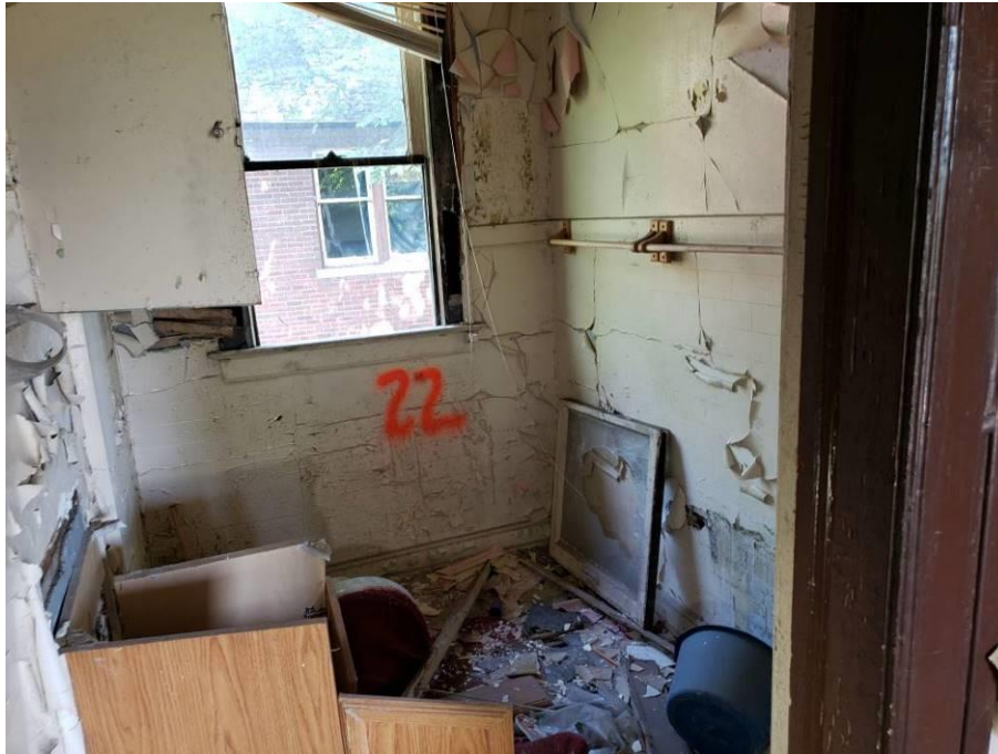
View of FS-22 (2 nd floor unit)
