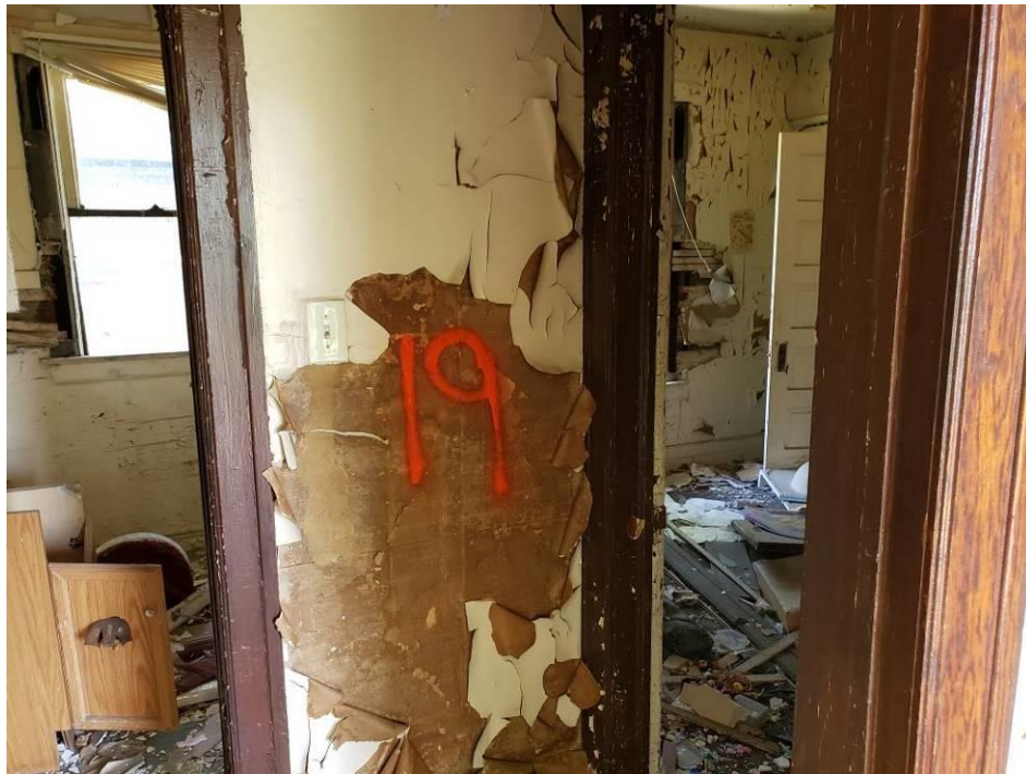
View of FS-19 (2 nd floor unit)
