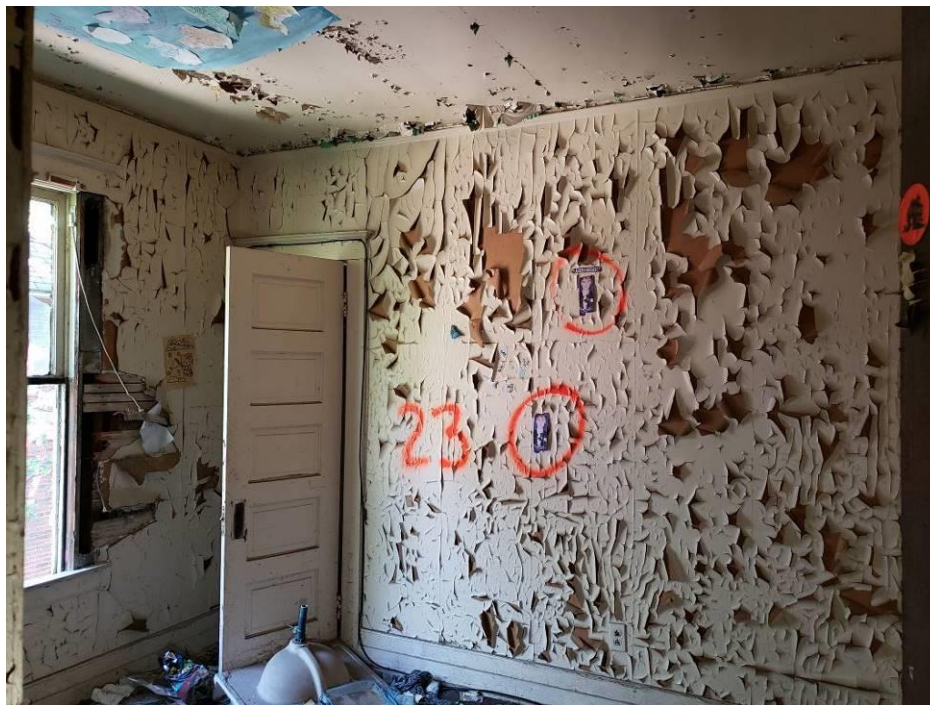
View of FS-23 (2 nd floor unit)
