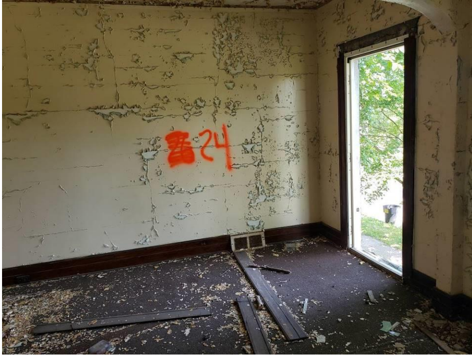
View of FS-24 (2 nd floor unit)
