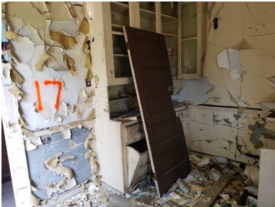
View of FS-17 (2 nd floor unit)
