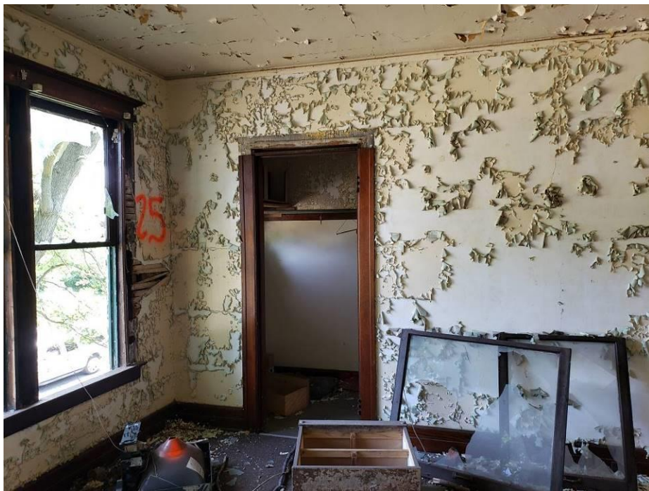
View of FS-25 (2 nd floor unit)
