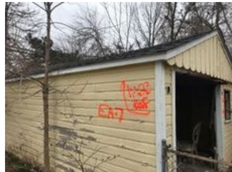
AS 11-1 Garage Roof Shingles
