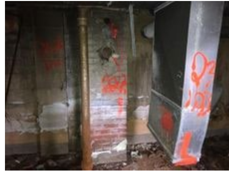
AS 22-1 Stack Cement
