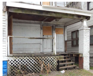
Porch rebuild needed
