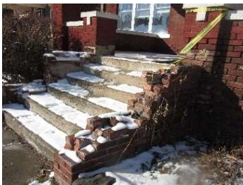
Collapsing porch wing wall
