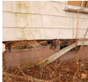
Rotted wall and trim board
