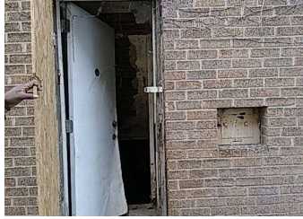
Door replacement needed
