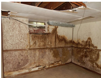
Evidence of water intrusion
