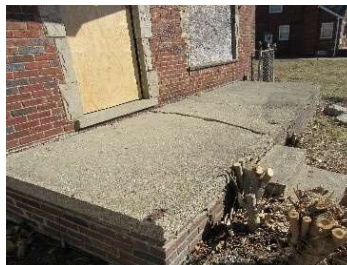
Cracked porch deck
