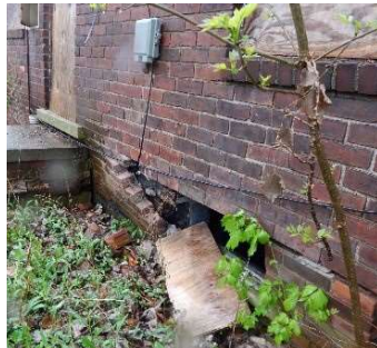
Failed exterior brick wall
