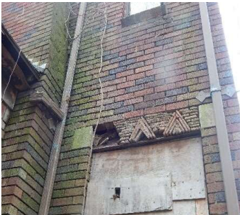
Missing brick above lintel
