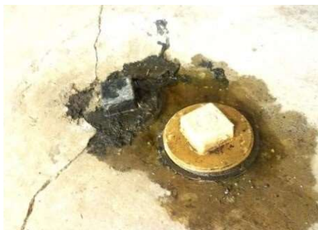
Leaking clean out plug
