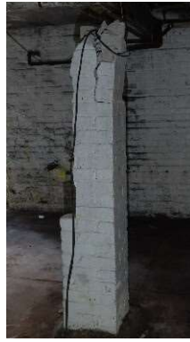
Failed brick column
