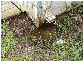
Pooling water near foundation
