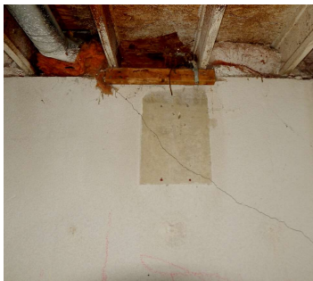
Cracked poured foundation
