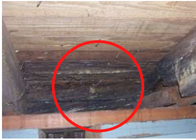
Rotted subflooring and joist
