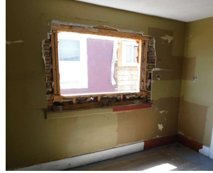
Window needs new install
