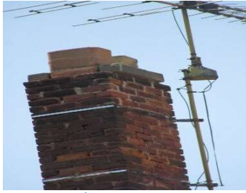
Missing chimney cap
