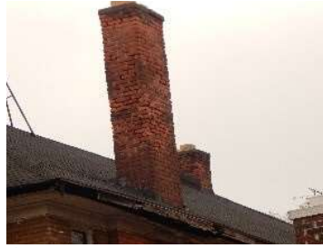
Open mortar joints
