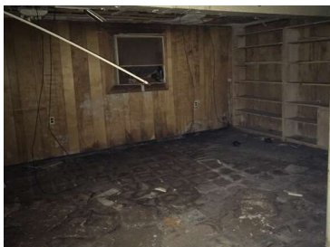
Evidence of previous flooding
