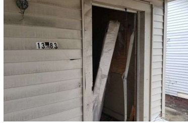
Missing door, damaged frame
