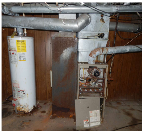
Water damaged furnace and water heater
